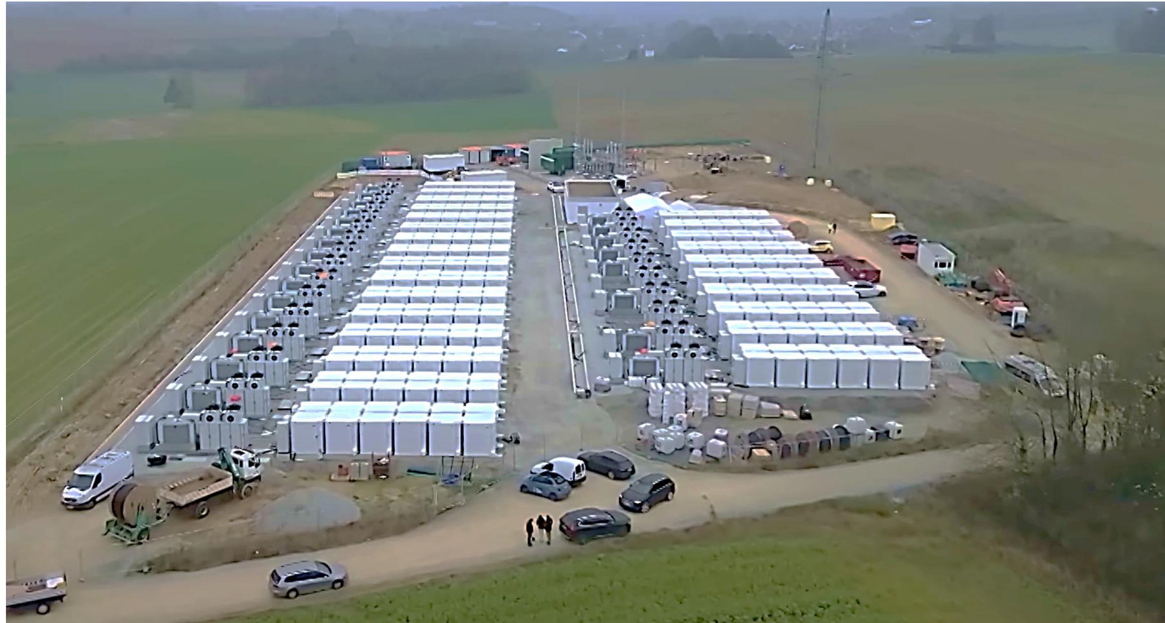
100 MW / 200 MWh BESS Wunsiedel (Bavaria)
